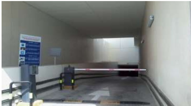
Traffic Barrier with Long Range Reader (ESAG Interiors Building–Karama)
